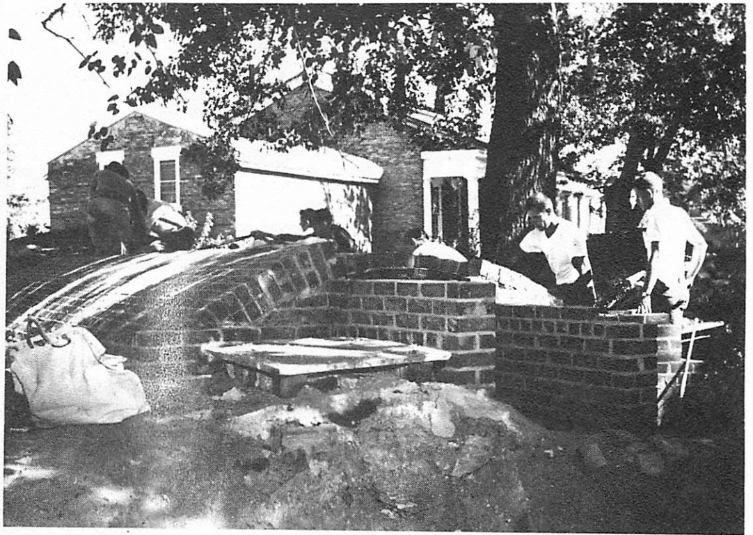
Restoration of the Root Cellar by Apprentice Bricklayers, Local 29, Bricklayers and Masons International Union
